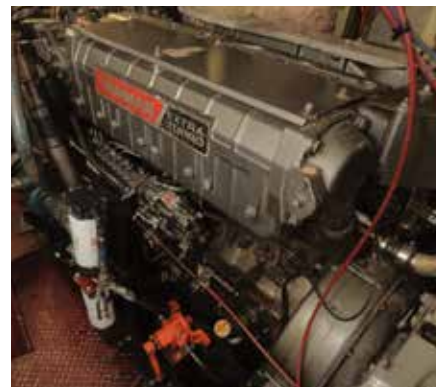
The ever reliable Yanmar 6HYM-ETE in the engine room.
